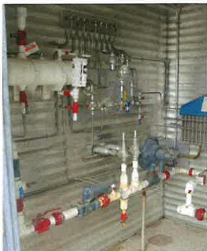
Interior of first type of RMO station.
