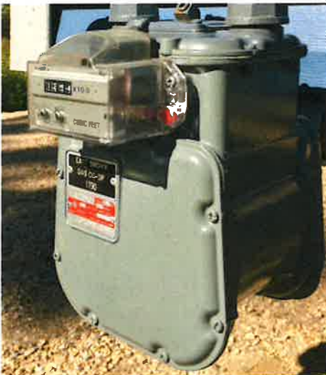
Example of a typical gas meter.
