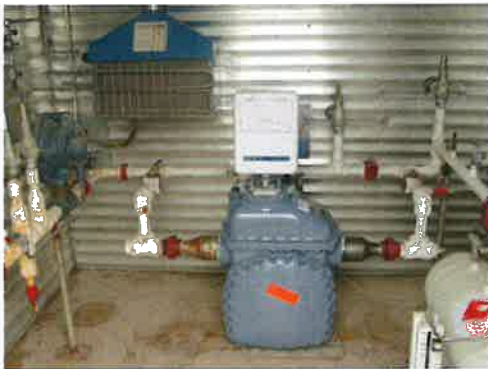
Interior of first type of RMO station.
