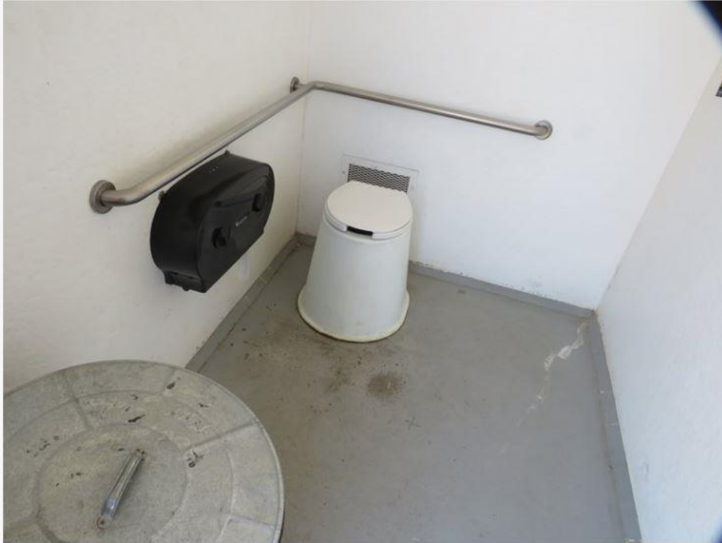
Sample interior of pedestal toilet on concrete floor, with accessible hand rails, spacious interior for ease of wheelchair access
