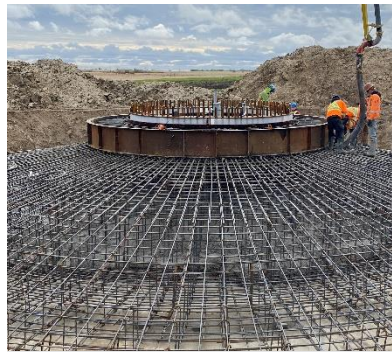
Getting ready to begin pumping concrete for the first wind turbine pour on May 22.
