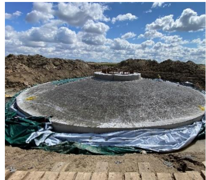
The first completed wind turbine foundation. Once the concrete cures, the foundations are backfilled leaving only the pedestal above the ground.
