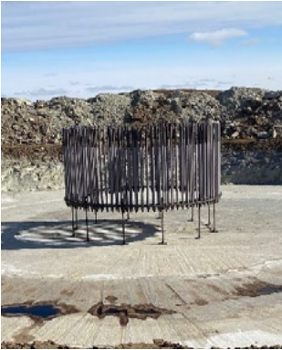
Bolt cages are assembled with steel rebar for the pedestal that supports the wind turbine’s steel towers as part of the foundation.
