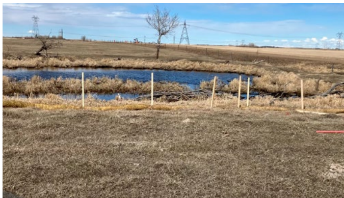
Wetland protection measures being put in place prior to cable crossing boring nearby and cable ploughing.
